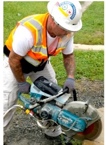
Applying water to the blade of a handheld power saw reduces the amount of dust created when cutting.
